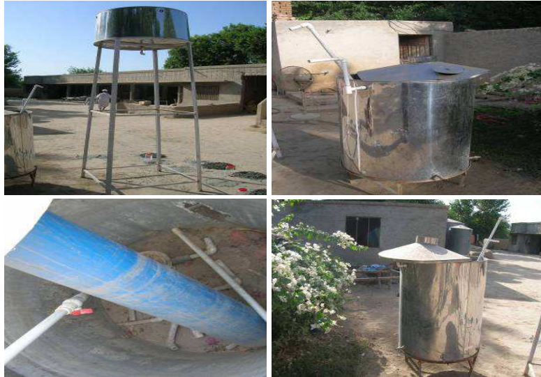
Figure 7. Damaged ARTs tanks which are non-functional and in dismantled conditions
